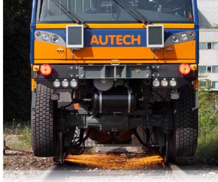
Camera-monitored track grinding unit for removing ripples, bumps, and rust from both sides of the track.
